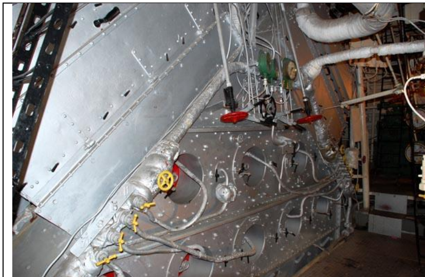
Front view of one of the boilers
